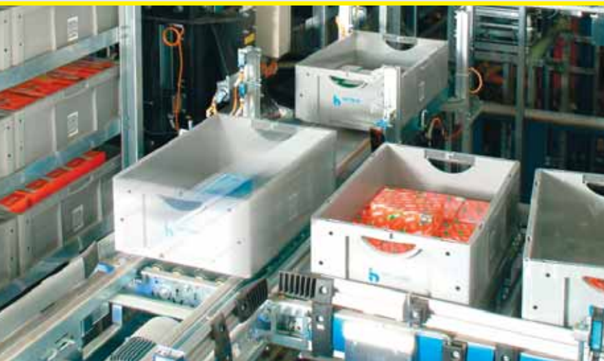
Conveyor system in front of miniload®
