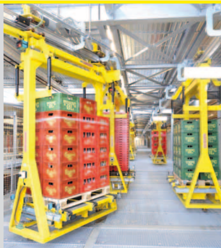
265 trolleys are located on the taxiing guide line of the electric Monorail between production and warehouse. Overall length 4 km.
