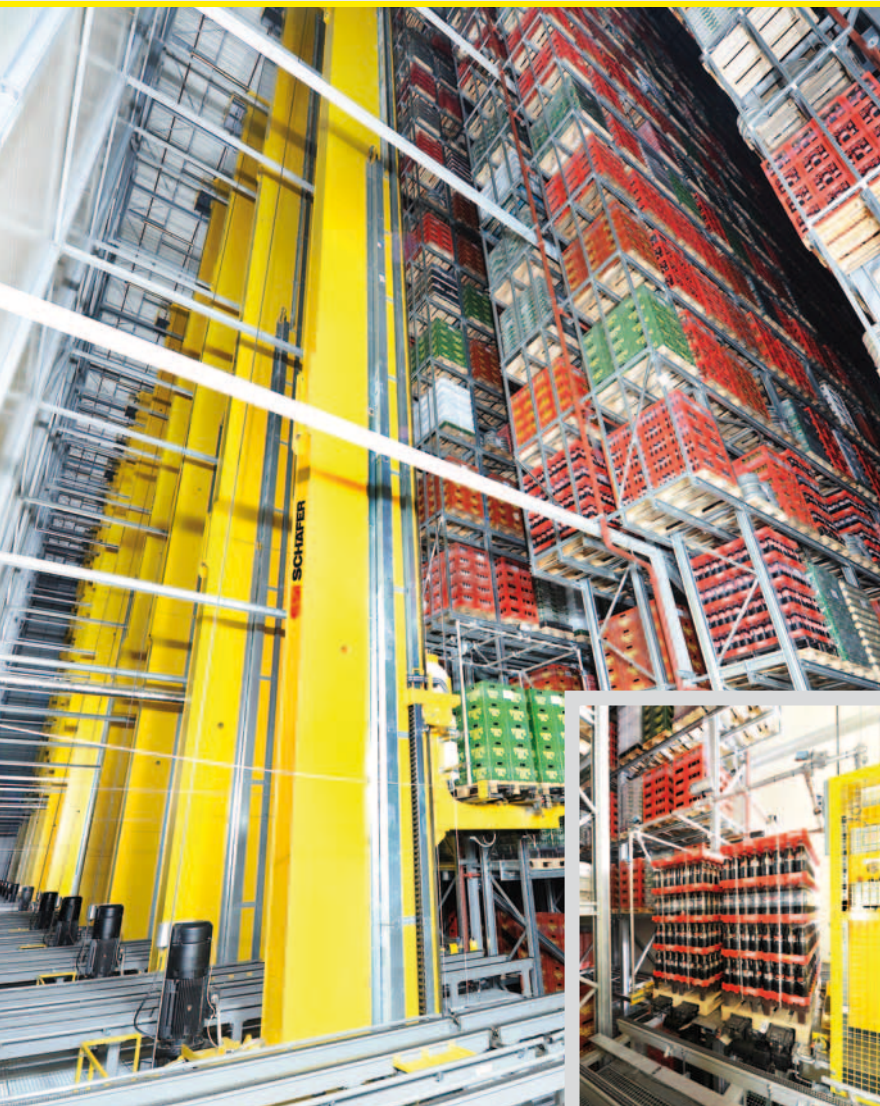
Pallets with beverages ready to be shipped are available in the 18 aisles of the 9,000 m 2 large HBW. Load acceptance with two double telescopic forks.
