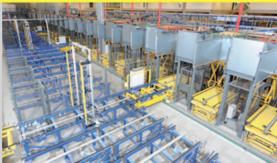
The lift tables are connected to the chain conveyor system via shuttle vehicles that run underneath the order picking platform
