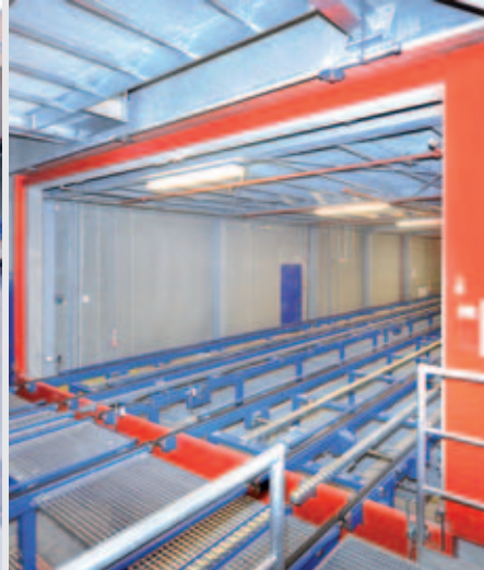
In case of emergency, fire gates seal off the conveyor line to the HBW
